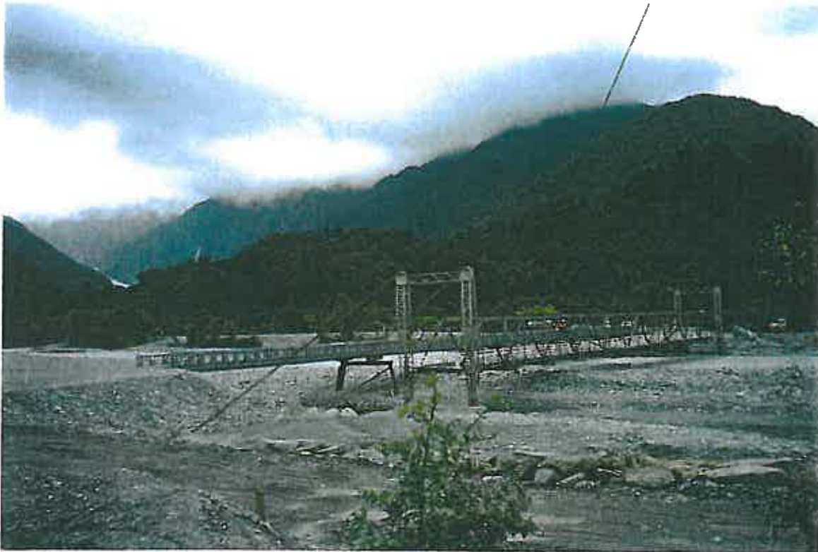
Figure 8.8 - The Waiho River at Franz Josef which has had a history of flooding and aggradation. The old bridge has had to be cut and lifted to maintain the waterway while a new temporary bridge has been put in immediately upstream for SH 6. This type of aggradation is likely in many other rivers draining the Southern Alps following an Alpine Fault earthquake.
